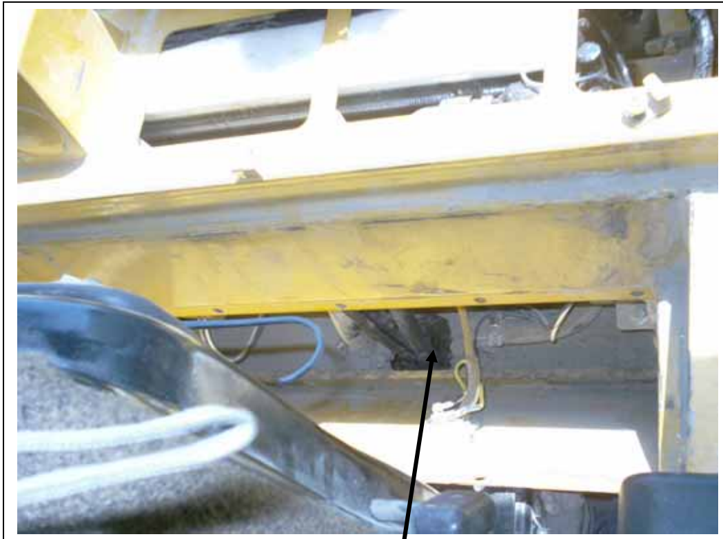
Seal opening with tar tape once the hoses are run into the cab
