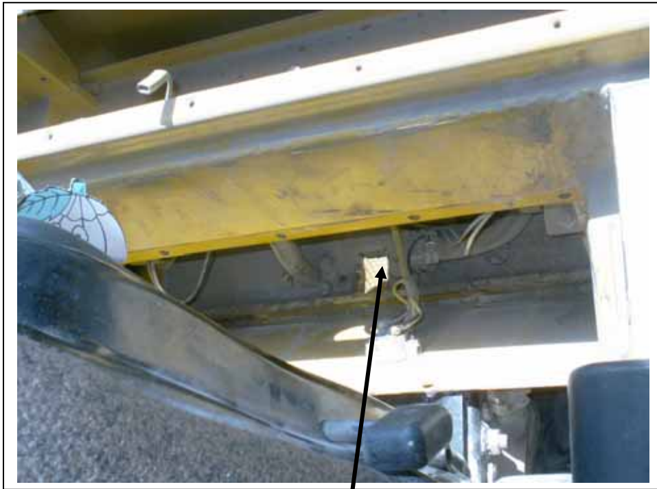
Drill, cut, chisel open this area to allow A/C hoses into the cab.
