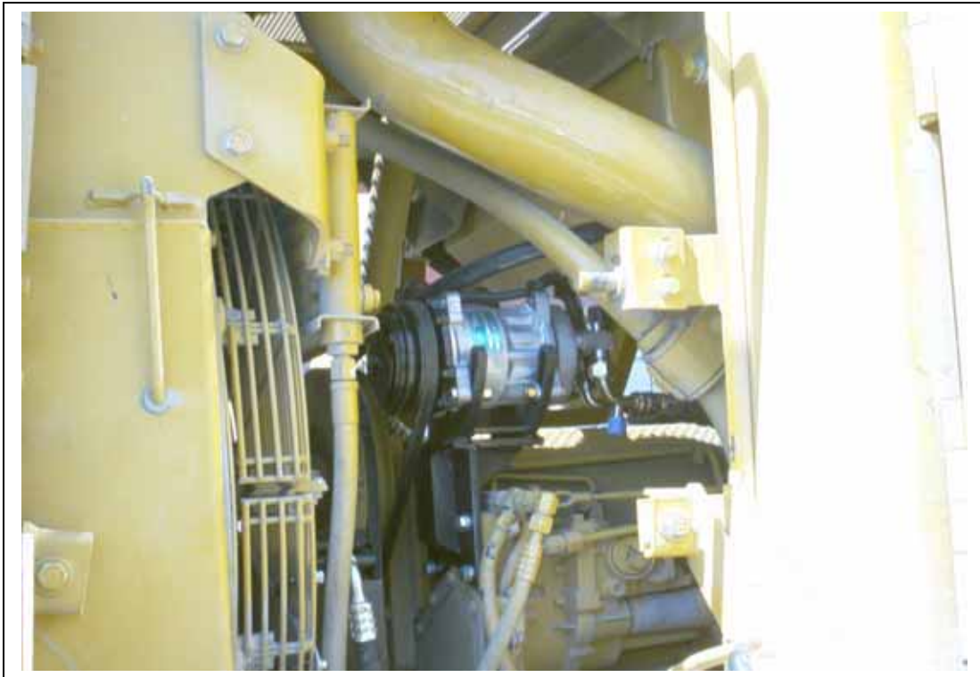
Compressor and mount in place
