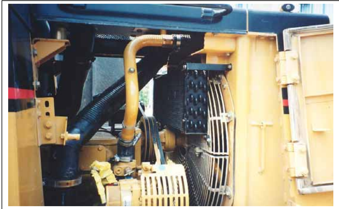
Left side of condenser mounted to fan screen
