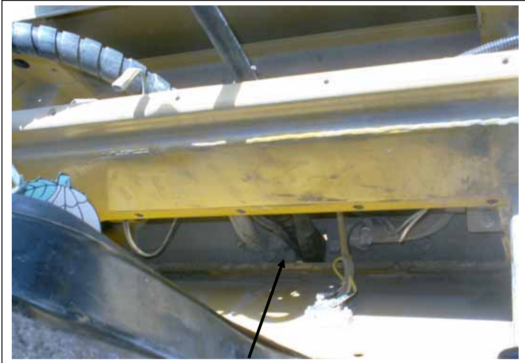
A/C hoses and wiring coming up through the floor of the cab.
